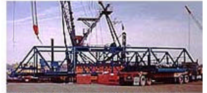
The freshly painted 100 foot transfer span sat on Boyer Barge's dock along with its head frame and towers (on the truck) waiting to be loaded by American Construction's large crane (background). The dock is less than 1/2 mile from Long's shop facility.
